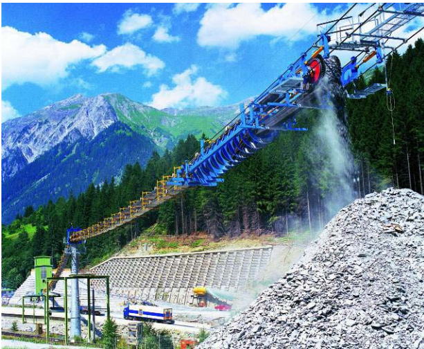
Figure 8. Fitting in the ropespan are the return/tension station, belt turning devices, re-rail track and track widener
