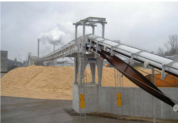
Figure 19. View from the loading station with belt turn-over section and conveyor track
