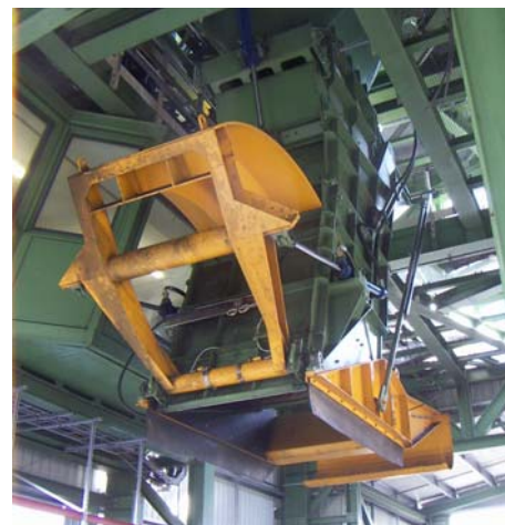
Figure 5. Installed load out spout inside the rail load out building
