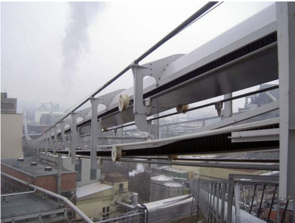
Figure 18. View from the discharge station on top of a tower back to conveyor track
