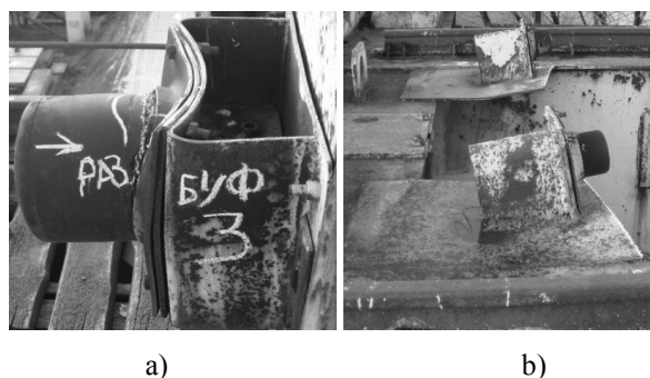
Figure 2. Damageability of bridge cranes' MC in the places of end buffers installment: a –end buffer installment bracket's MC; b- ES installment brackets' MC
