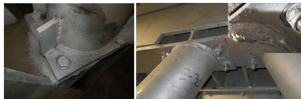
Figure 10: Cracks of vertical bracings
