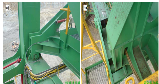
Figure 5: The final design of the counterweight boom supporting system: front a); rear support b)
