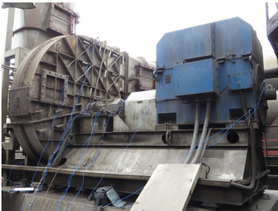
Figure 13. View of the placement of vibrations sensors on the ventilation unit
