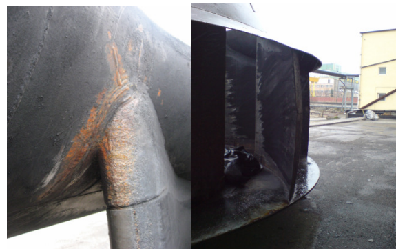
Figure 12. Fracture of fan impeller, large deformation of blade
