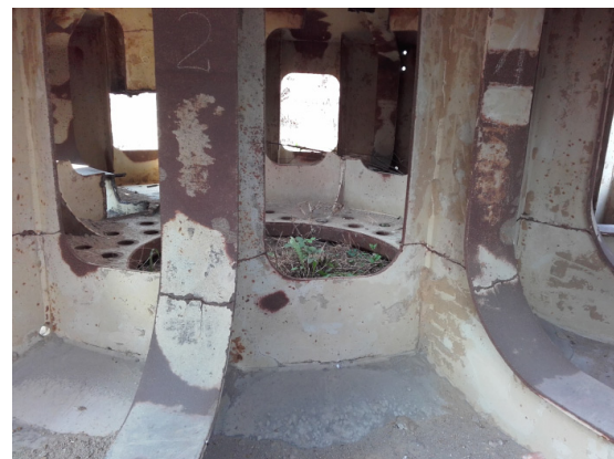
Figure 6. Failure of the bucket wheel structure
