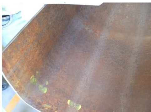
Figure 1. Cleaning the area of application of strain gages from metal oxides is the first step.
