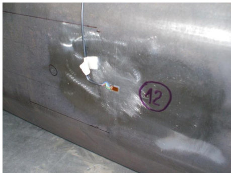
Figure 28: Monitor the plates so as to immediately highlight instability effects.
