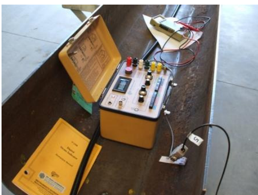
Figure 19: Check the resistance in the various connections by means of a tester.
