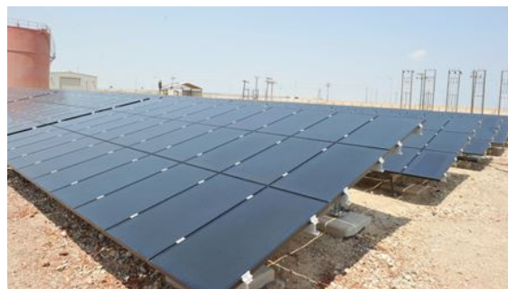
Figure 9. Photo of a 500 kW installed capacity PV power plant in Farasan Island near Gizan, Saudi Arabia
