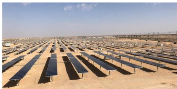
Figure 7. Layla solar photovoltaic power plant, Layla, Al-Aflaj, Saudi Arabia [16]
