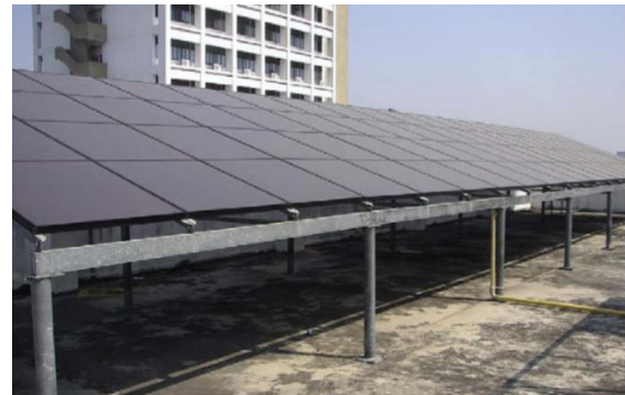
Figure 12. Building-integrated photovoltaic system of 4.872kW rated capacity in Thailand [74].
