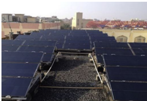
Figure 16. Roofmounted BIPV system at Sawda School tested under harsh environmental conditions in Kuwait [105]
