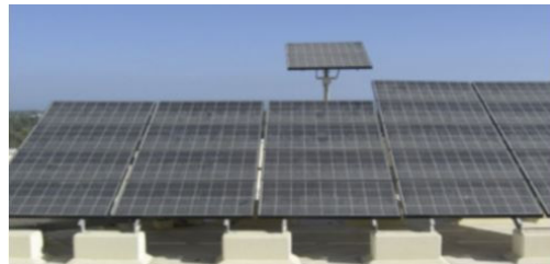
Figure 17. A 1.4 kW BIPV system installed on a building at Suhar University, Oman [111]
