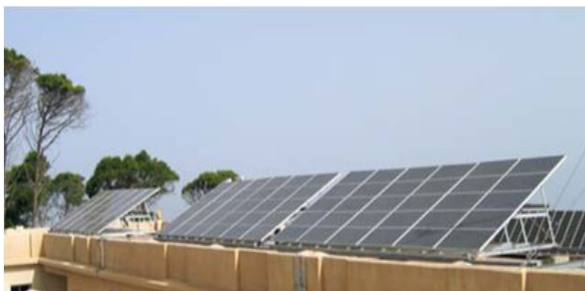
Figure 5. Roof mounted monocrystalline technology BIPV demonstration plant in Algeria [22]
