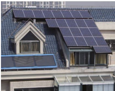
Figure 10. 3kW BIPV system in Shanghai, China [47]
